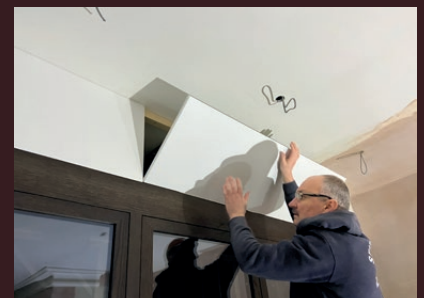
False wall with access panel created to disguise climate control
